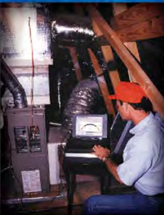
A professional Aeroseal technician will monitor the duct leakage in your home
