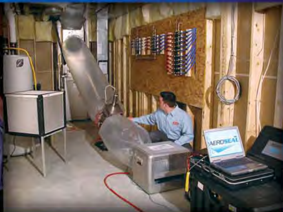
Aeroseal software allows the technician to accurately measure the duct leakage in your home
